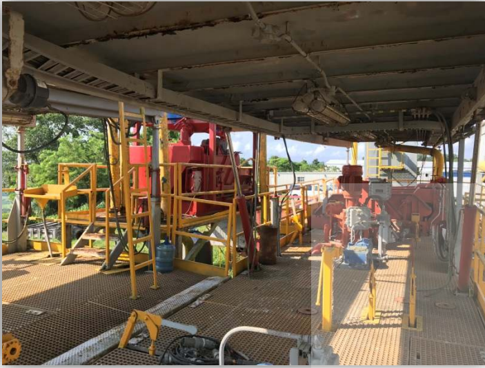
MUD TANK SECOND
