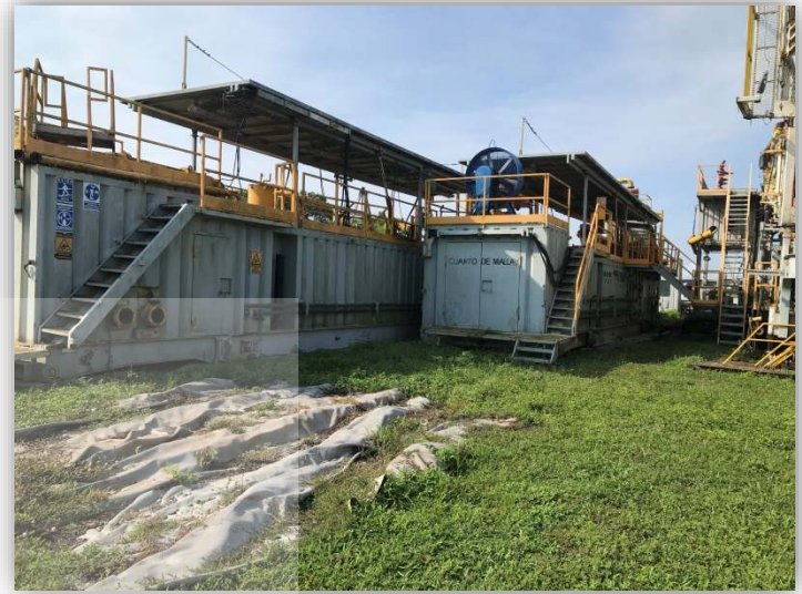
SUCTION MUD TANK
