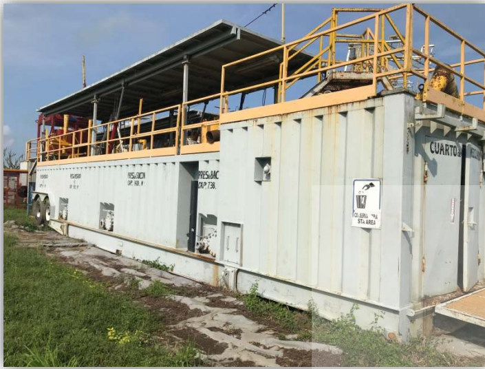
SUCTION MUD TANK
