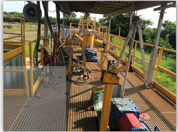
MUD TANK SUCTION
