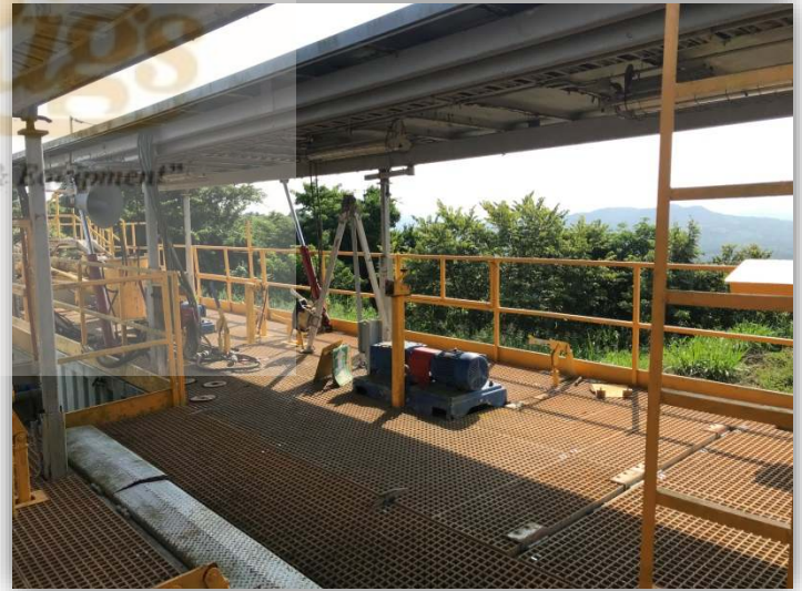
MUD TANK SUCTION
