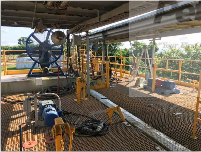
MUD TANK SUCTION
