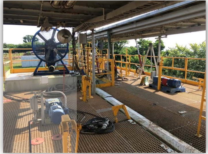
MUD TANK SUCTION
