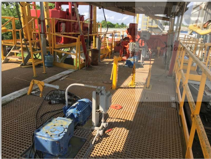
MUD TANK SECOND
