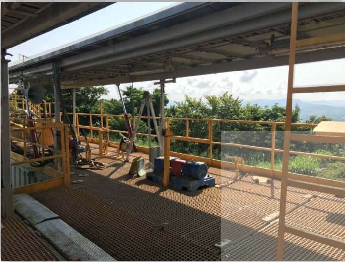
MUD TANK SUCTION
