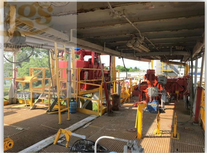
MUD TANK SECOND
