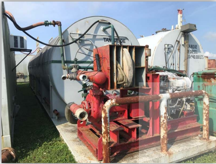
WATER TANK & FIRE PUMP
