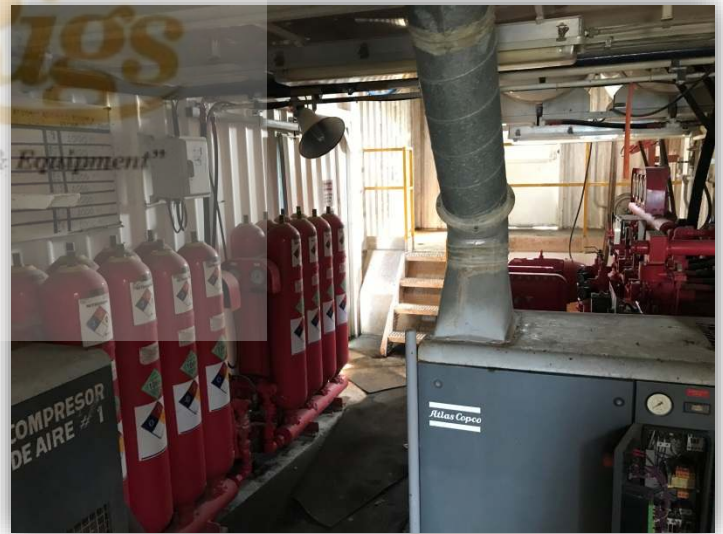
COMPRESSOR MAIN & ACCUMULATOR
