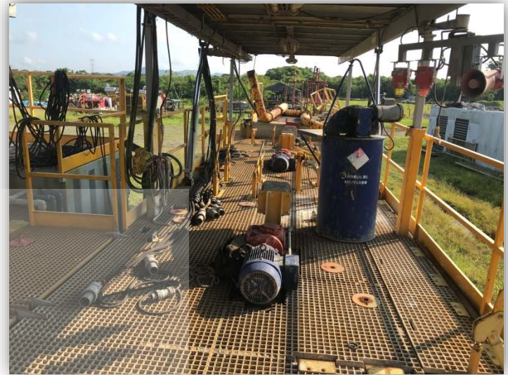
SUCTION MUD TANK
