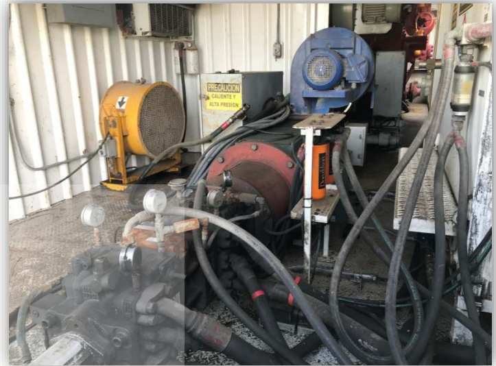
HYDRAULIC POWER UNIT
