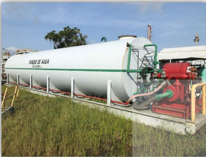
WATER TANK & FIRE PUMP
