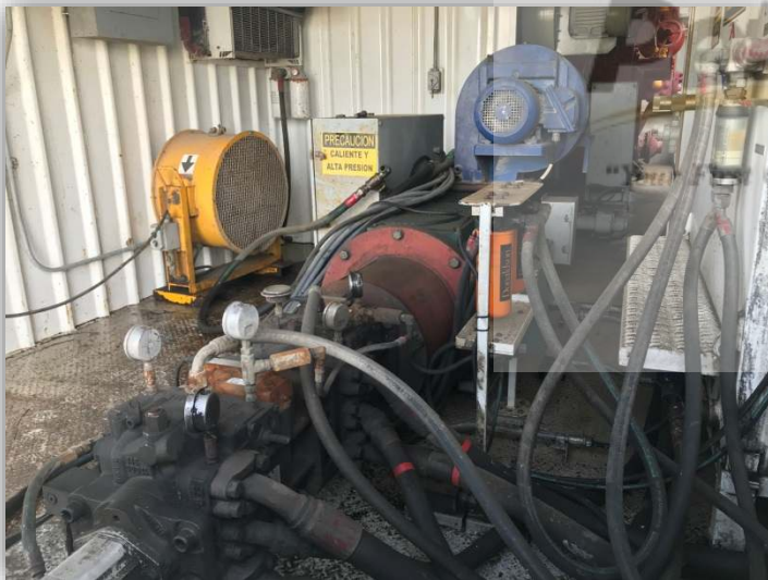
HYDRAULIC POWER UNIT
