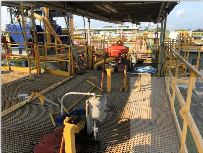
MUD TANK SECOND
