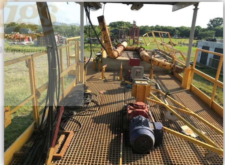
SUCTION MUD TANK
