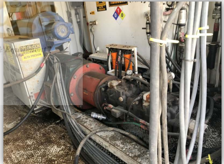
HYDRAULIC POWER UNIT
