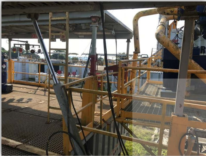
SUCTION MUD TANK
