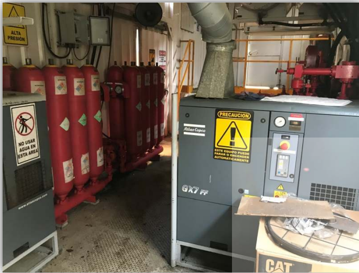
COMPRESSOR MAIN & ACCUMULATOR
