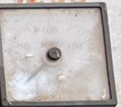
DRAWWORKS BRAKE COOLING WATER
