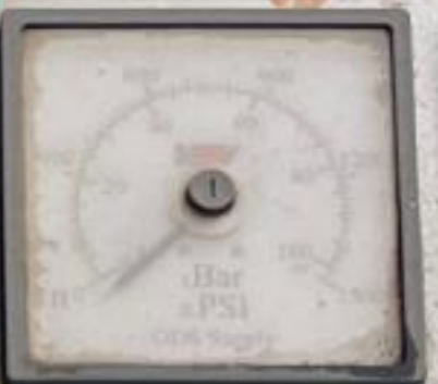
ODS SUPPLY PRESSURE
