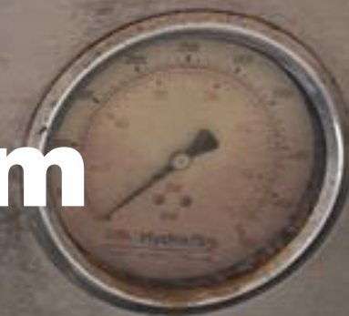
INJECTOR MOTOR PRESSURE
