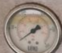
BOP SYSTEM PRESSURE
