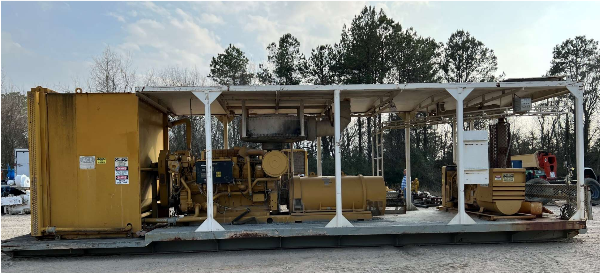
GEN HOUSE w/CAT 3512B S/N# 4AW01433 ARR# 174-4950 HRS: 45391 KATO GENERATOR S/N# 18315-13 1365 KW 1200 RPM
