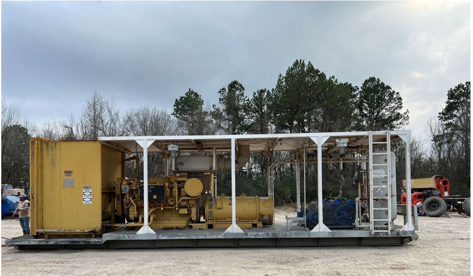
GEN HOUSE w/CAT 3512B S/N# 4AW01395 ARR# 174-4950 HRS: 44696 KATO GENERATOR S/N# 7865-04 1365 KW 1200 RPM
