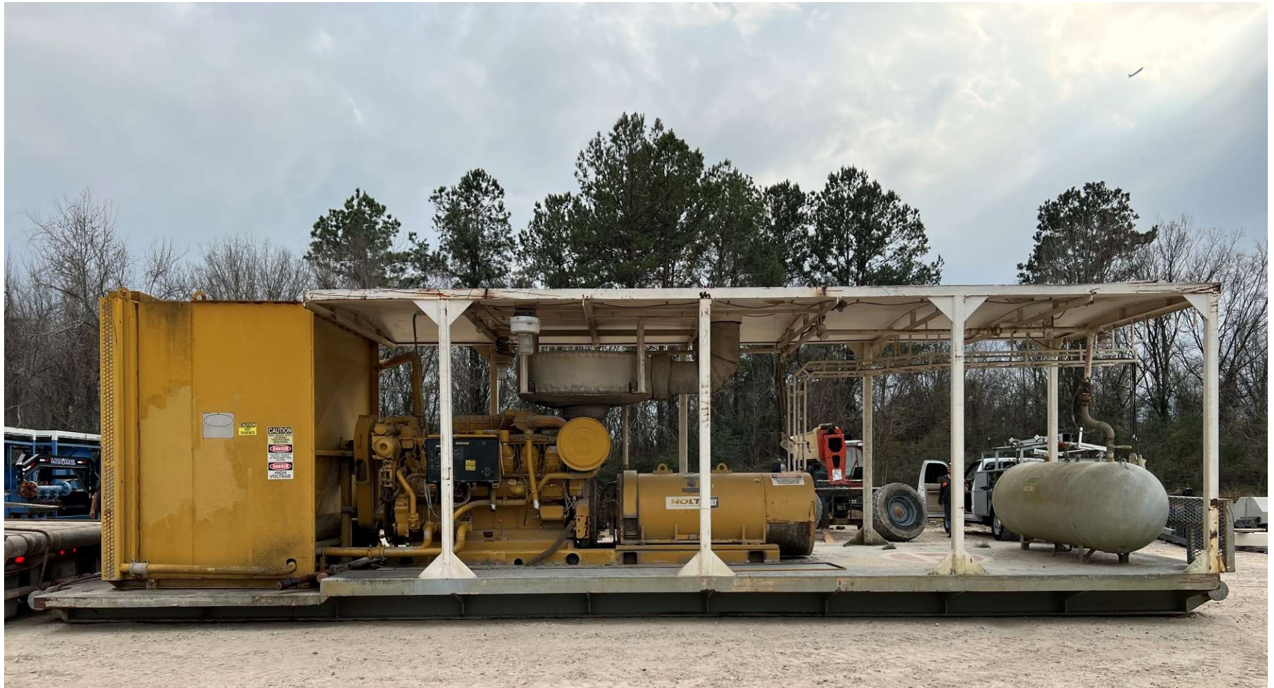
GEN HOUSE w/CAT 3512B S/N# 4AW01429 ARR# 174-4950 HRS: 45499 KATO GENERATOR S/N# 16862-04 1365 KW 1200 RPM
